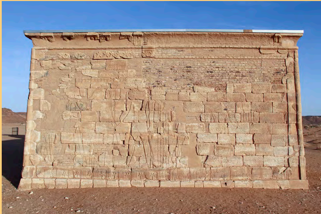
Colour fig. 5: Section of missing plaster on the outer west wall of the Apedemak Temple (photo: Cornelia Kleinitz).
